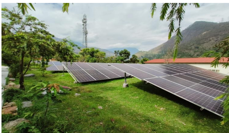
Fig. 23.6: 50KW Solar Power Plant under State Project by UREDA
